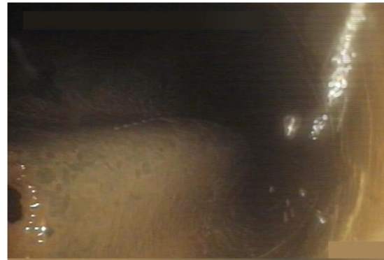
Figure 1: The buckling shape of a collapsed casing with external concrete support 1 .
