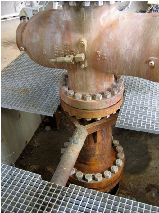
Figure 4: The expansion spool and master valve of the wellhead of well HE-46 (figure: Heimir Hjartarson).
